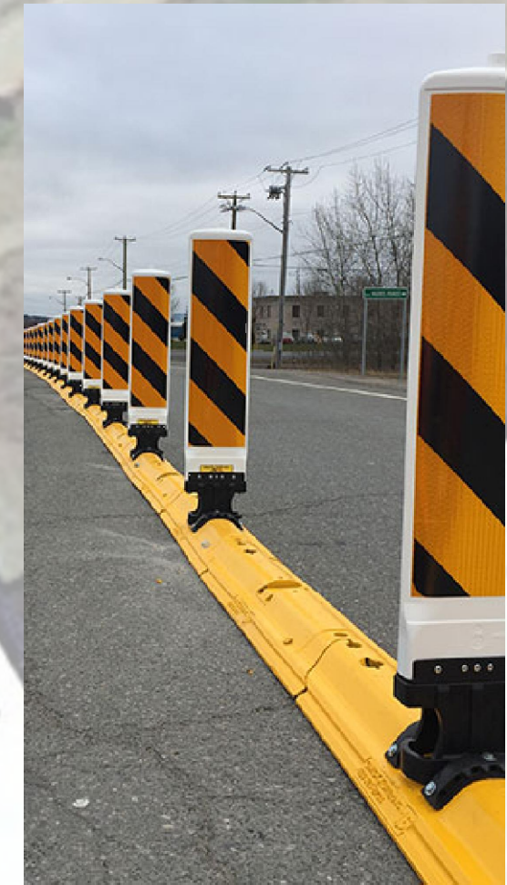
PHASE 1 - INSTALLATION OF QUICK KURBS AT MIDDLE SCHOOL NORTH SIDE CROSSING ON US-12. PHASE 2 WOULD INSTALL PERMANENT CURB WITH MDOT APPROVAL AFTER TRIAL PERIOD.
