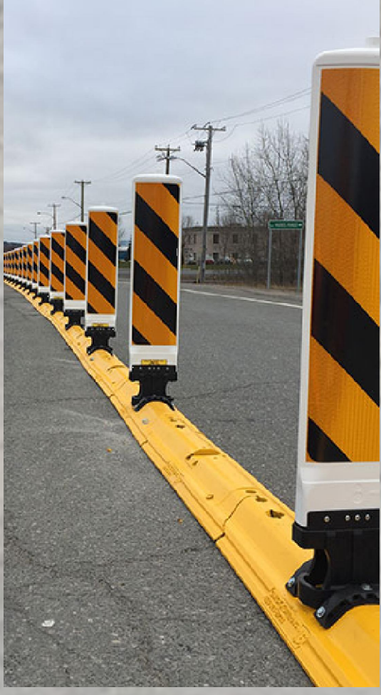
PHASE 1 - INSTALLATION OF QWICK KURBS AT TRAIL CROSSING ON US-12. PHASE 2 WOULD INSTALL PERMANENT CURB WITH MDOT APPROVAL AFTER TRIAL PERIOD.
