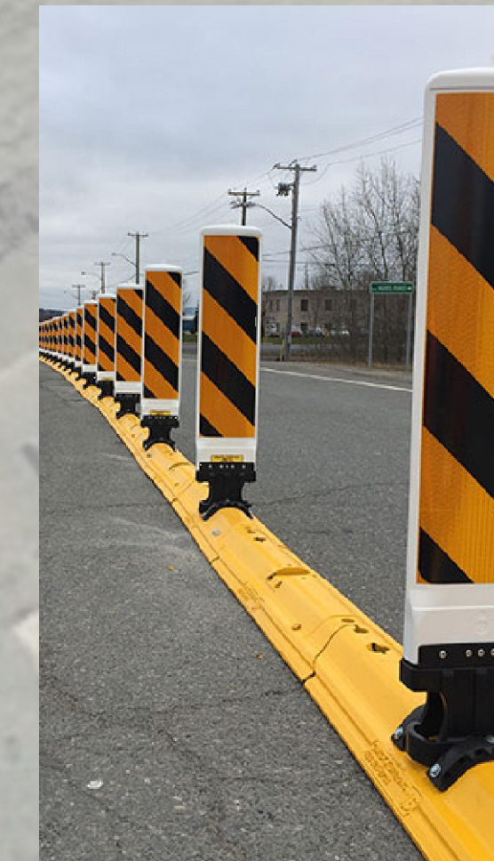
PHASE 1 - INSTALLATION OF QUICK KURBS AT MIDDLE SCHOOL NORTH SIDE CROSSING ON US-12. PHASE 2 WOULD INSTALL PERMANENT CURB WITH MDT APPROVAL AFTER TRIAL PERIOD.
